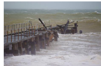
Port Rickaby jetty destroyed in wild weather
