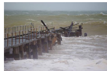
Port Rickaby jetty destroyed in wild weather
